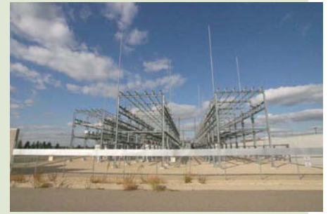
A substation at 28th Avenue and American Boulevard.
